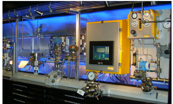
Sampling Condition Systems
